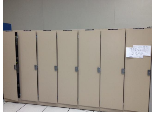
Figure 12 Train Control & S&C Modem Racks
