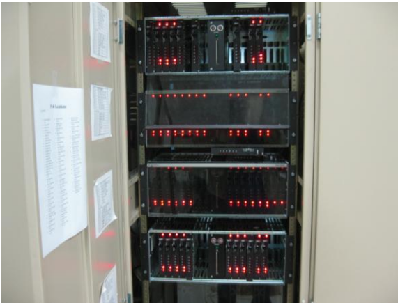
Figure 8 Front View of Modem Communication Rack
