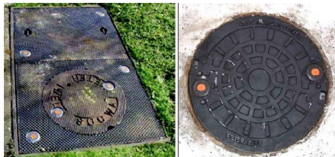
FIGURE 4 Utility Manhole Cover Locks
