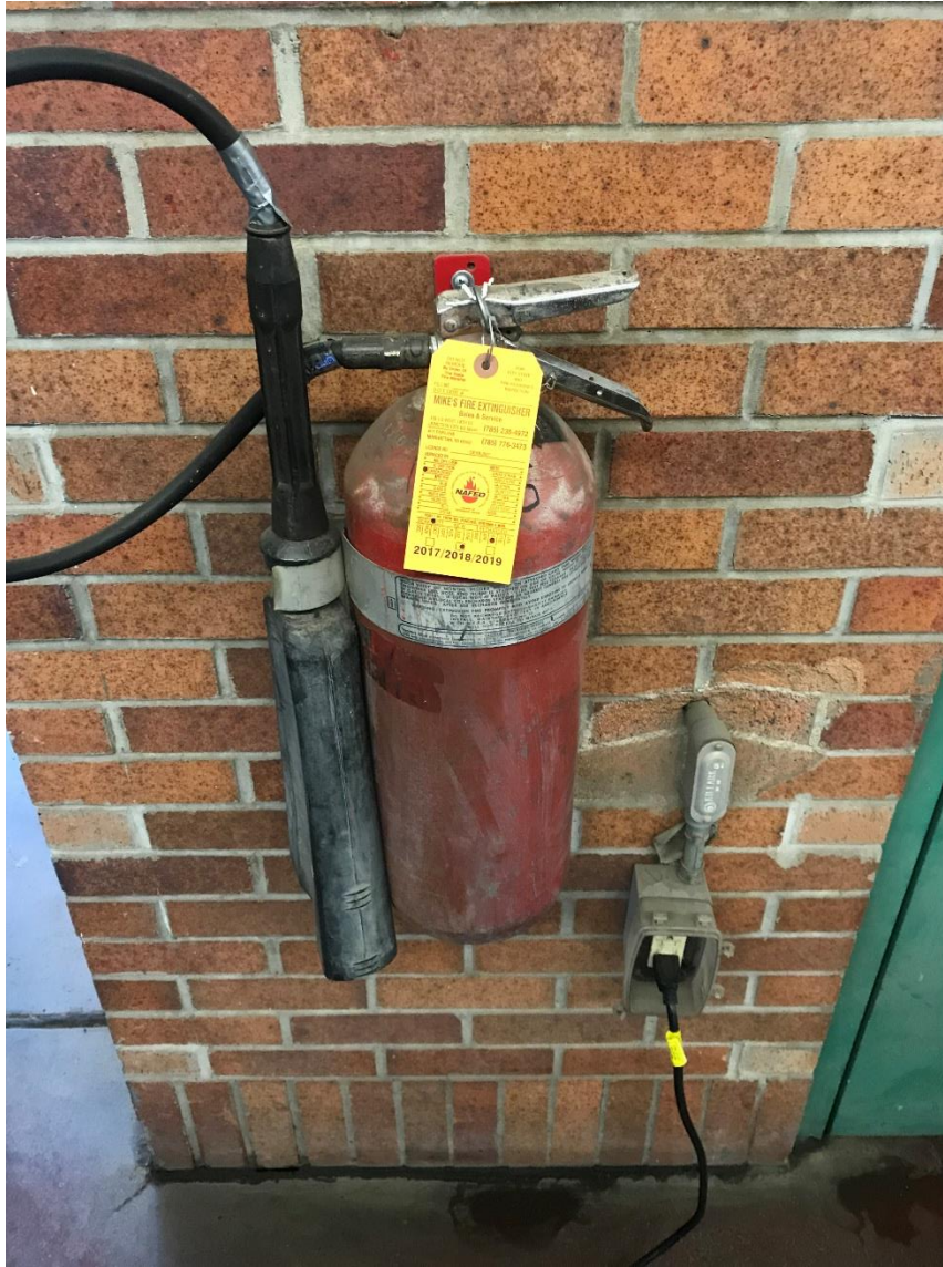
Figure 3: OCCK, Inc. Fire Extinguisher (Photo: TranSystems)
