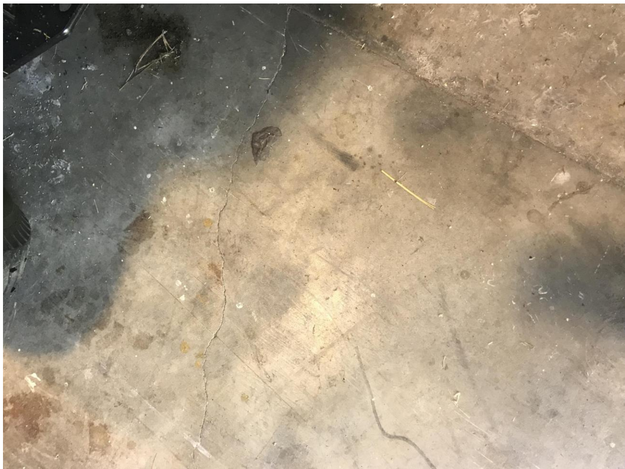
Figure 2: Maintenance Facility Floor with Cracks, SEK-CAP (Photo: Groundswell Consulting)
