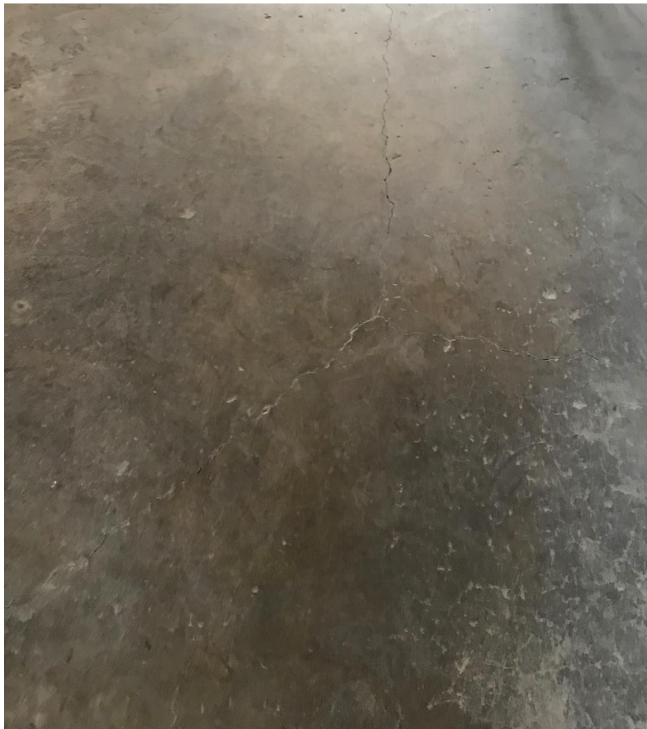
Figure 2: OCCK, Inc. Floor Cracking Example (Photo: TranSystems)
