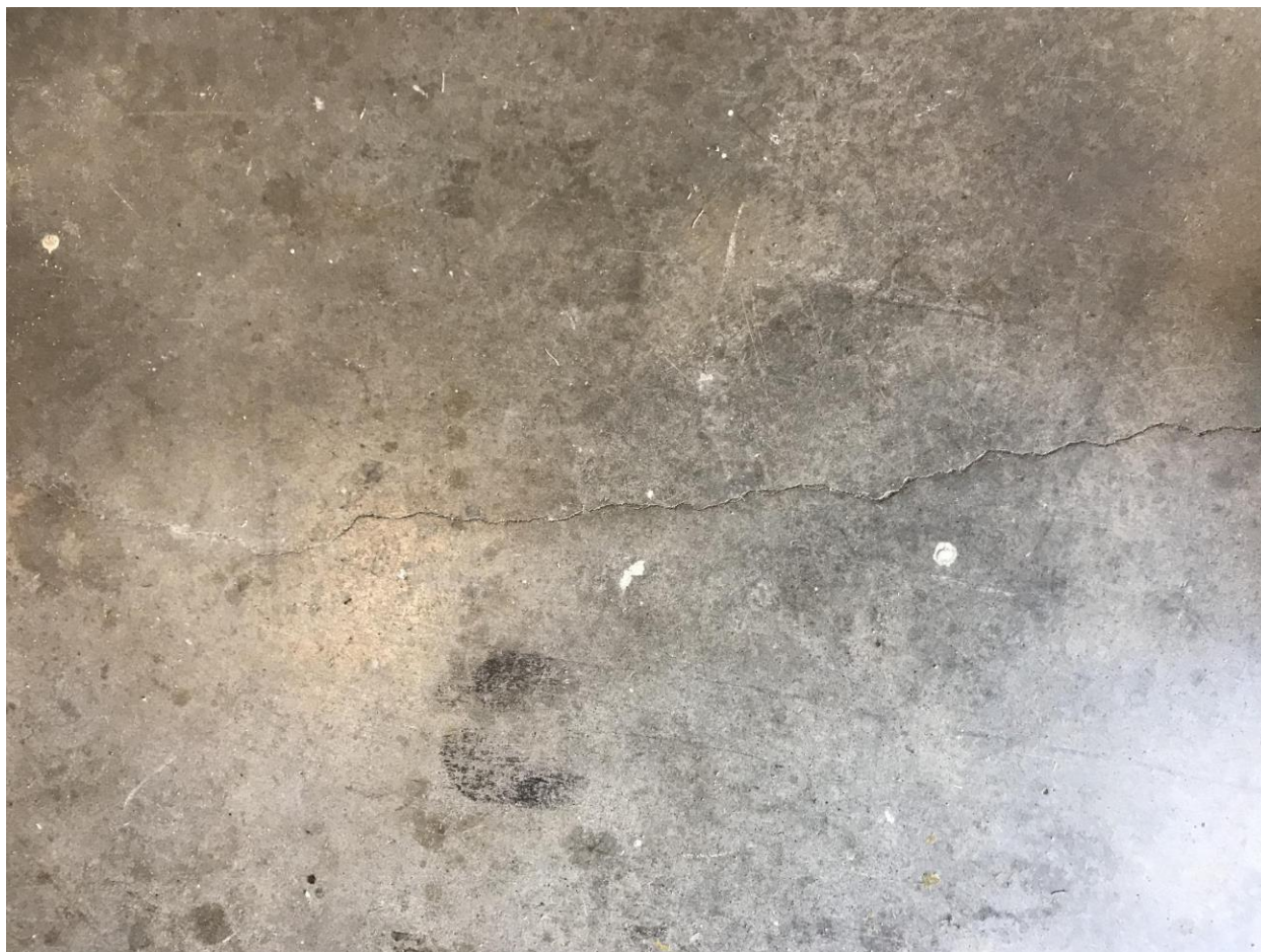
Figure 3: Maintenance Facility Floor with Cracks, SEK-CAP (Photo: Groundswell Consulting)
