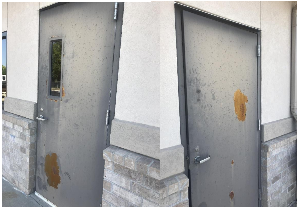
Figure 4: Wear on West-facing Doors, SEK-CAP Administrative Facility (Photo: Groundswell Consulting)
