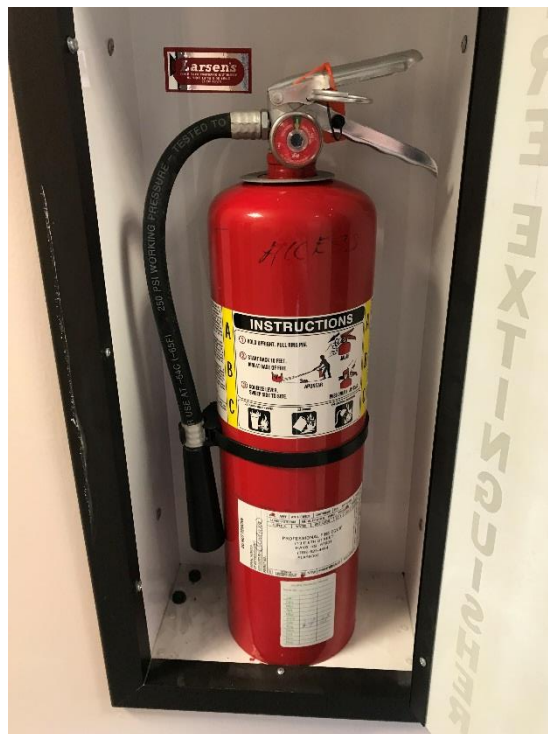
Figure 2: Access Transportation, DSNWK Extinguisher (Photo: TranSystems)
