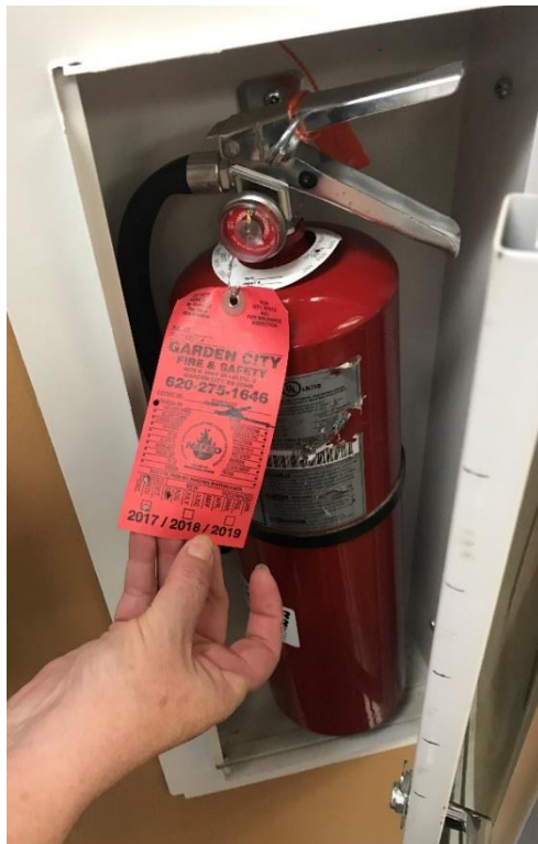
Figure 2: Finney County Fire Extinguisher (Photo: TranSystems)
