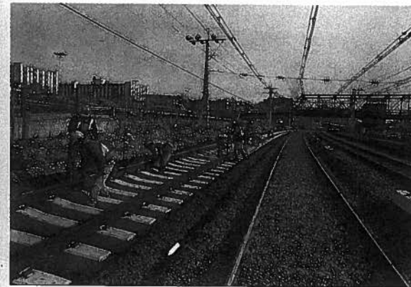
Track workers at the MTA Metro-North Railroad in New York City pursue their never-ending task of making sure the roadbed and track are in good repair.
