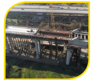
There are 30 active construction sites spanning 119 miles across five counties: Madera, Fresno, Kings, Tulare and Kern.
