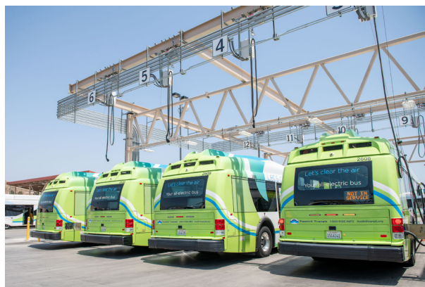
FIGURE 3 —Conductive charger with overhead reel plug-in dispenser (courtesy Foothill Transit)
