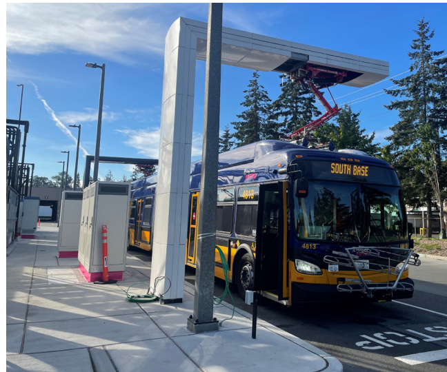
FIGURE 2 —Conductive charger with pantograph, King County Metro facility (courtesy Lisa Jerram)
