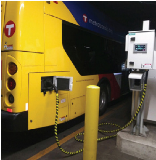
FIGURE 1 —Conductive charger with ground mount plug-in dispenser (courtesy Metro Transit)
